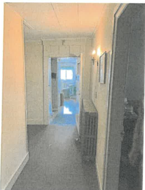
Photo 18. A view from within Section B, looking south toward the West Kitchen Wing. This doorway, which would likely have originally been an exterior entry, has a transom and a shouldered surround.
