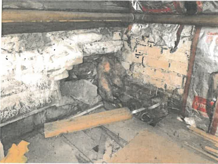
Photo 25. The same attic-level view of the intersection of the stone wall of Section A (left) and brick wall of Section B (right).
