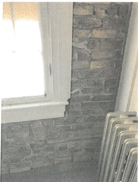
Photo 22. On the second story, the west wall of the small central bedroom of Section B affords a view of one of the brick walls that defines this section.
