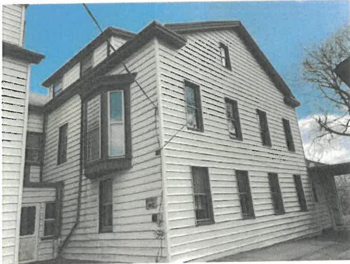
Photo 7. The west elevation of the two-story ell towards the south end of Villa St. Joseph.
