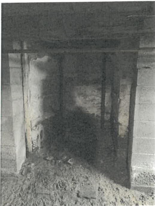
Photo 32. An arched feature at the south end of the basement of Section A, likely a hearth support.
