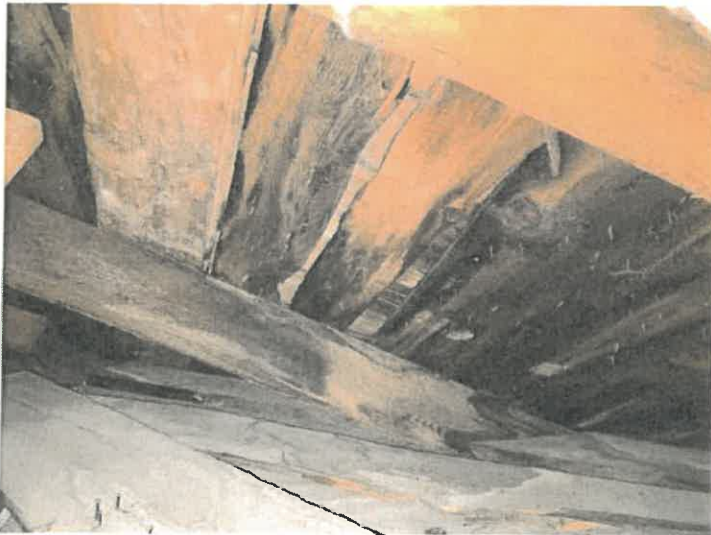
Photo 26. The same location as above, showing the rafters and sheathing that appear to represent the structure of the roof that connects Section B to Section A; this was laid over the original rafters and sheathing of Section A (at bottom).
