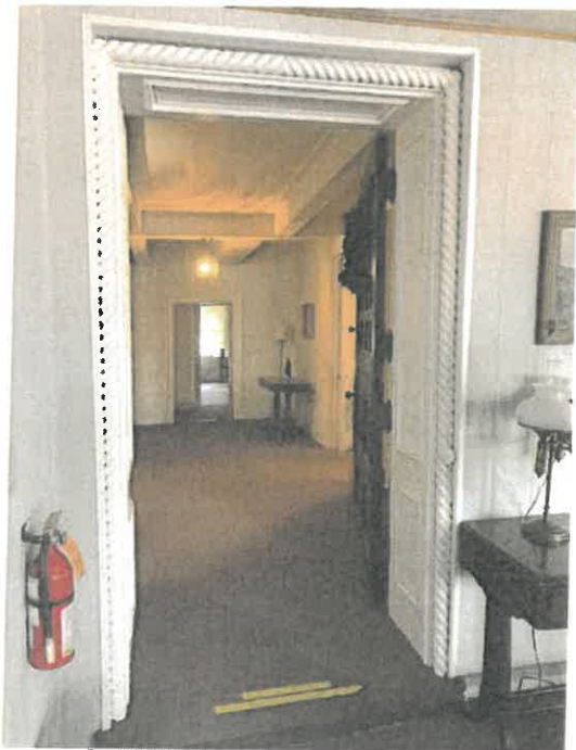
Photo 14. The same doorway, looking west from the Enclosed Porch to the Hall within Section A.
