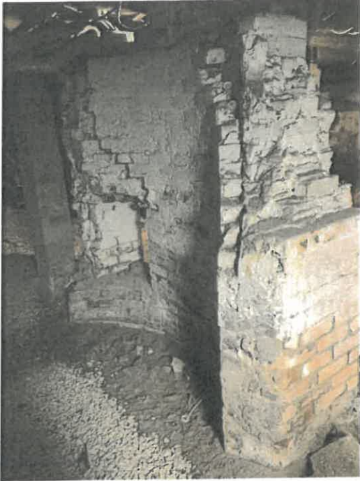
Photo 31. A curved brick feature within the basement of Section A, possibly the remnant of a cistern.
