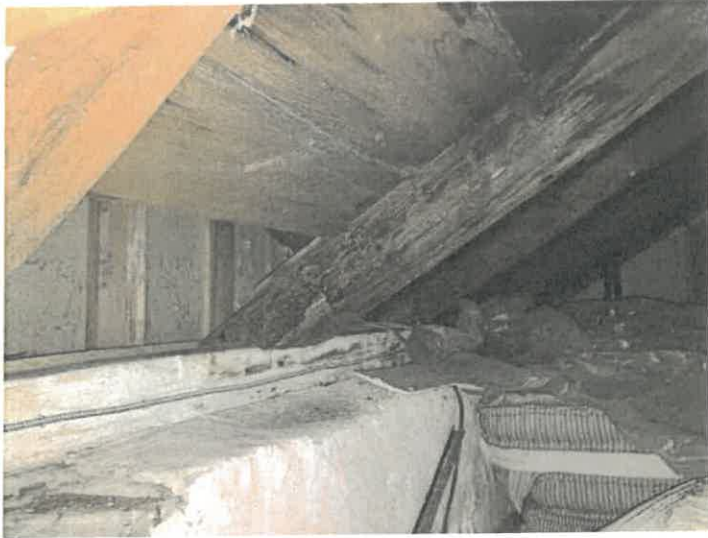
Photo 27. Another glimpse into the roof structure of Section A is found in another small closet in the upper story of the building. Shown here is sheathing atop rafters seated on a timber wall plate set on the top of the stone wall of this section of the house.
