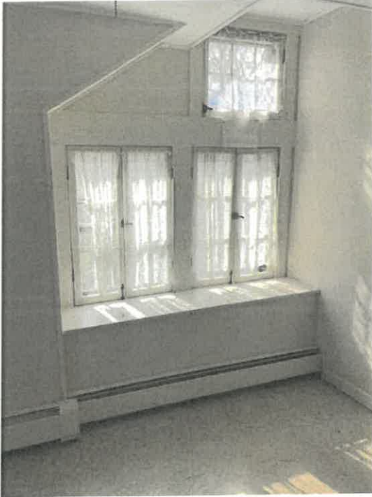
Photo 23. At attic story level, the south (gable end) wall of Section A within a bedroom at the southeast corner of the building.
