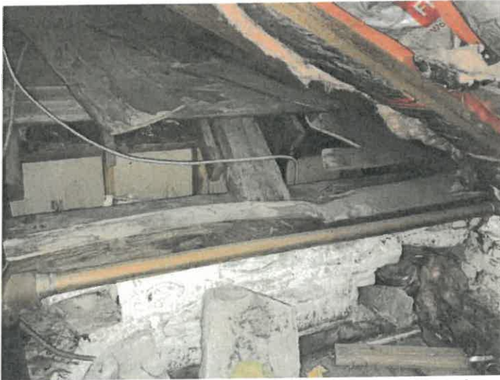
Photo 24. A small closet at attic story level at the junction of Sections A and B provides a window into the construction of these two sections of the building. At center is the upper portion of the stone wall of Section A with the timber wall plate and earlier roof structure. To the extreme right, the intersecting brick wall of Section B is visible and a later roof structure above.
