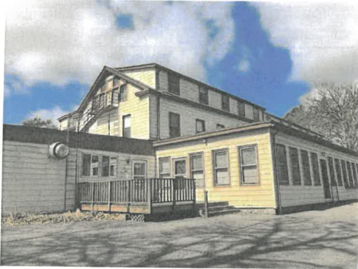
Photo 1. The south and east elevations of Villa St. Joseph. The east kitchen wing is visible on the left. The former porch is visible at the right.
