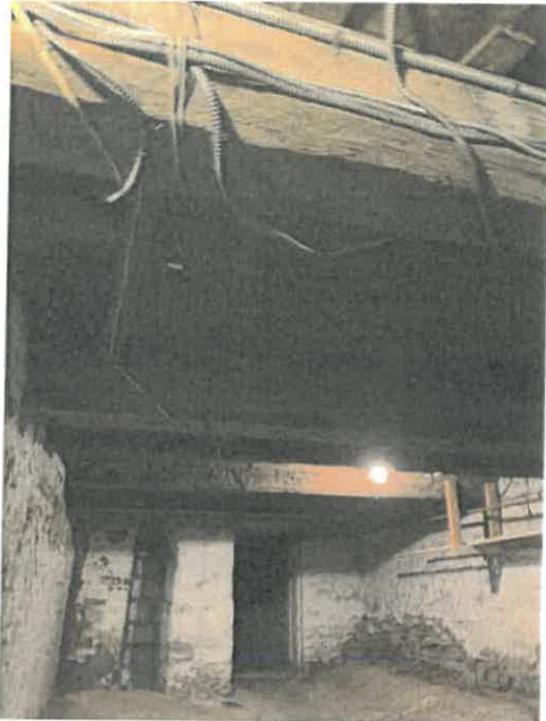
Photo 29. A view within the basement of Section A, showing the stone foundation walls, a brick partition to left, and large hewn beams.
